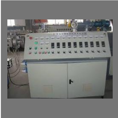
Extrusion Control Panel
