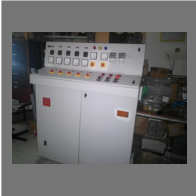
EXTRUDER CONTROL PANEL
